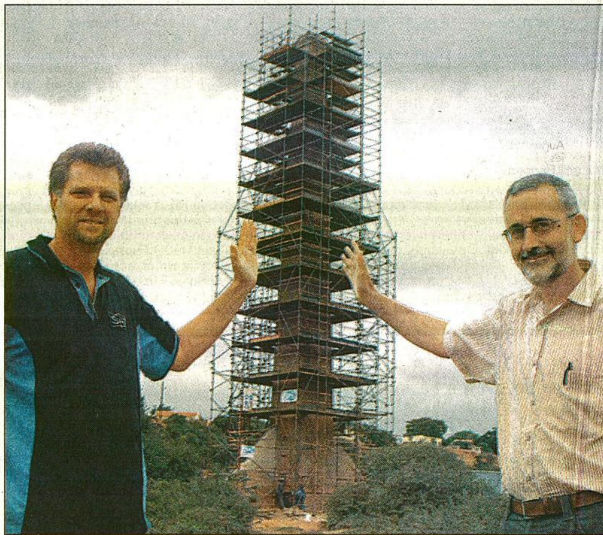
DESPATCH BEACON . . . Contractor Pieter Theunissen (left) and Despatch Museum chairman and former town clerk Attie Pretorius are two of the role players, together with the Nelson Mandela Bay municipality and Ivo Huisman Engineers, involved in the restoration of the historic Despatch chimney. Picture: FREDLIN ADRIAN
